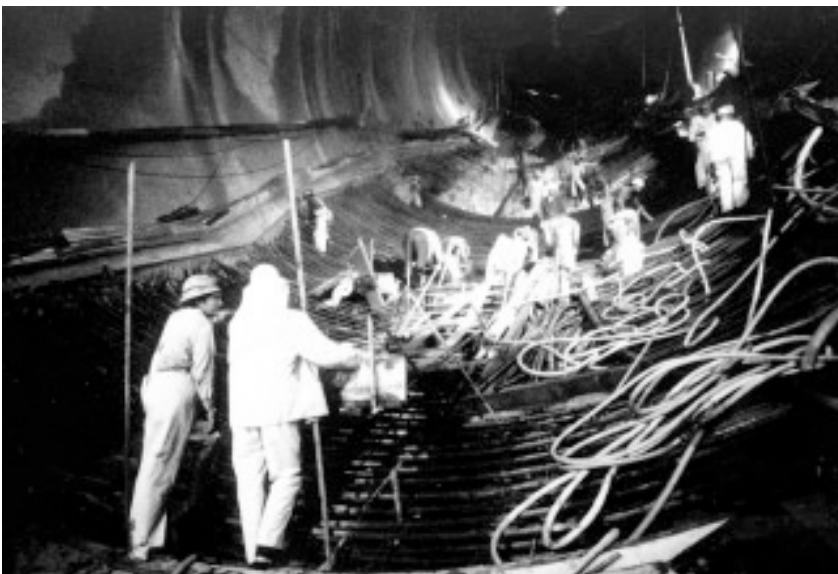
Figure 9 Photographs showing damage to spillway after 1983 flood (BOR).
